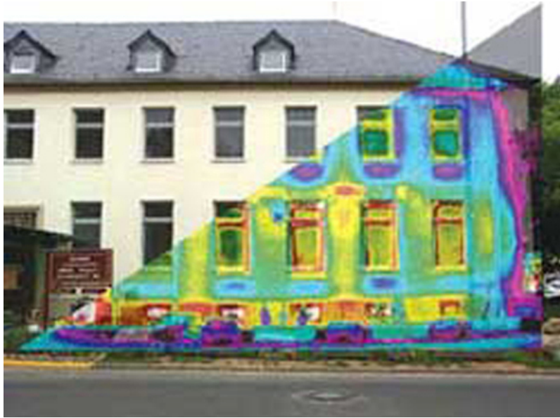
Figure 1.32 A thermograph of part of a building shows temperature variations, indicating where heat transfer to the outside is most severe. Windows are a major region of heat transfer to the outside of homes. (credit: US Army)
